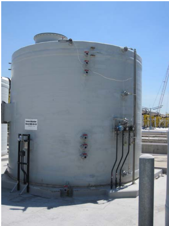
Figure 5 - North Control Building Carbon Adsorber
